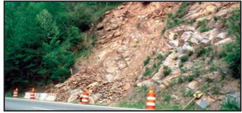
Figure 18. Rockfall near Gatlinburg, Tenn.
